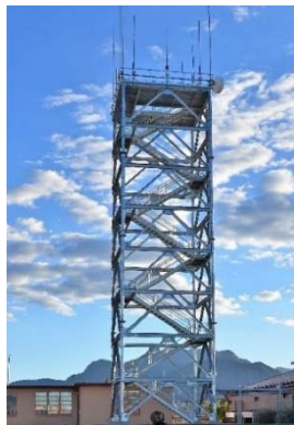
80' communications tower (available up to 100')
